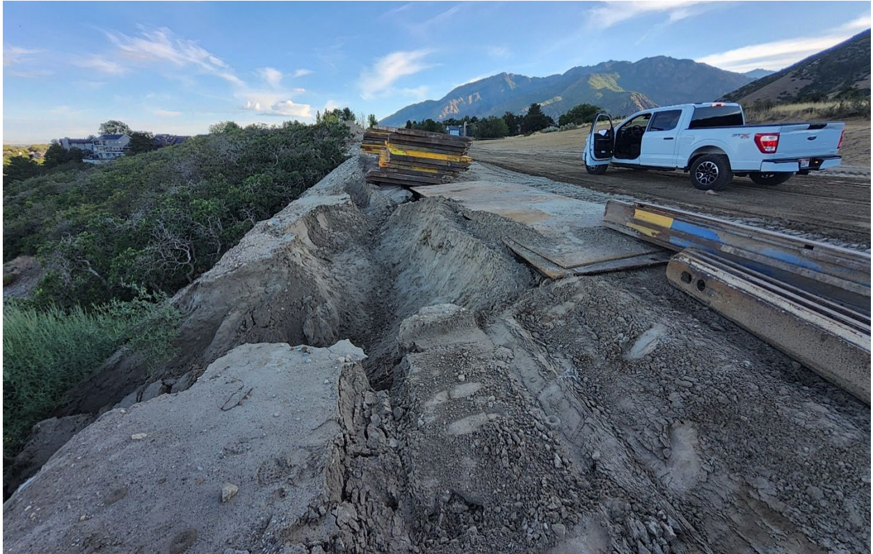
A rain storm on August 13 caused erosion and filled the SLAR with water and mud; the damage was quickly resolved.
