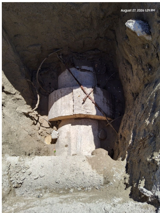
The LCC was exposed in Deer Creek Road.
