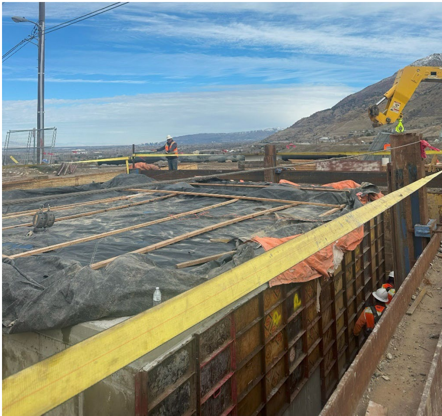
The CC-1 vault in Ft. Union Blvd. has a roof...the CC-1 vault is now fully enclosed. Preparing to backfill and connecting the CC-1 pipeline with the vault in May.
