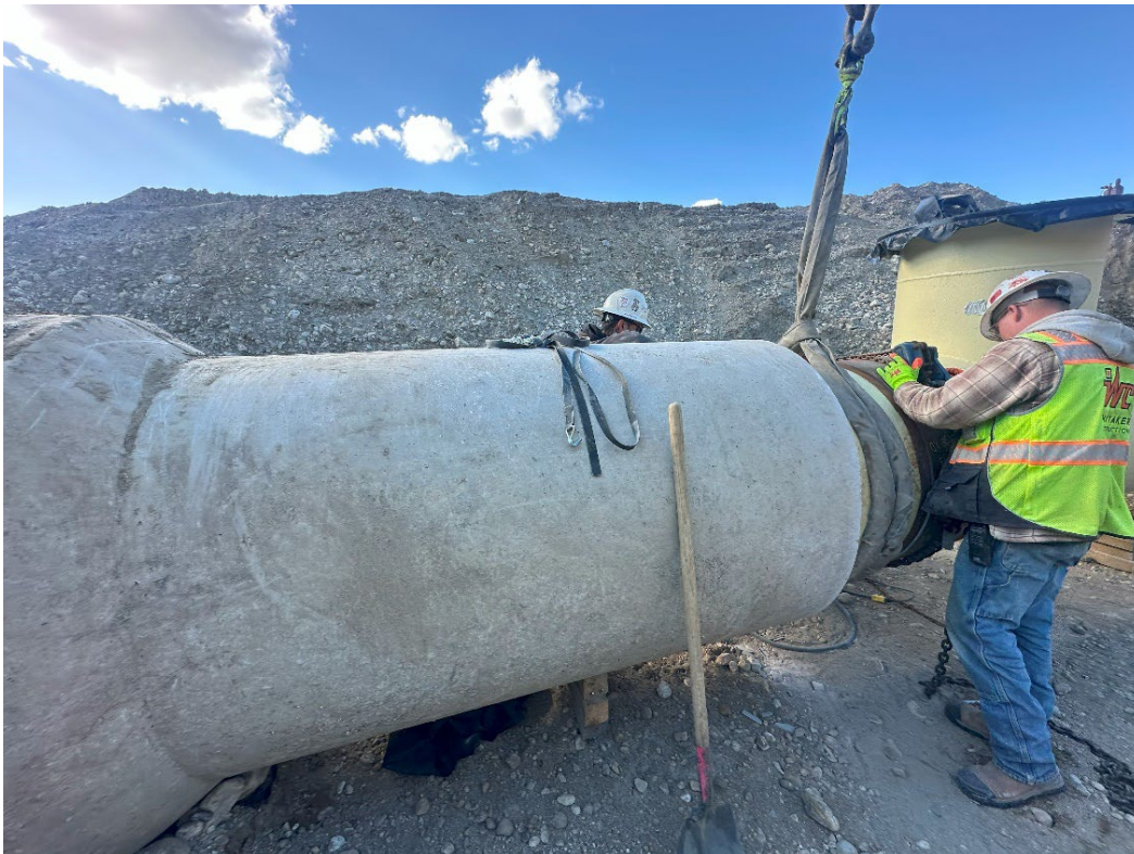
Out with the old, in with the new...connecting the new 36-inch steel LCC replacement (yellow pipe) with the old, original LCC concrete pipe near the 10 MG reservoir.
