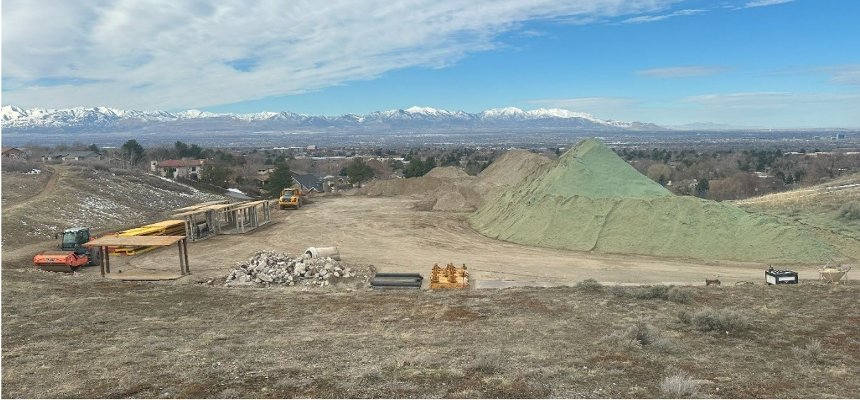
Nice and tidy...the large construction staging area at the 10 MG reservoir site. Piles of material have erosion control applied to prevent blowing sand and dust (green tint), trench shoring systems to the left, and old concrete that was removed in front.
