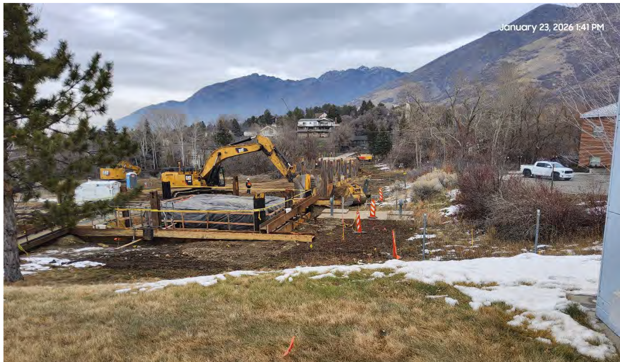
The SLAR pipeline is being installed west of the LCWTP Administration Building.
