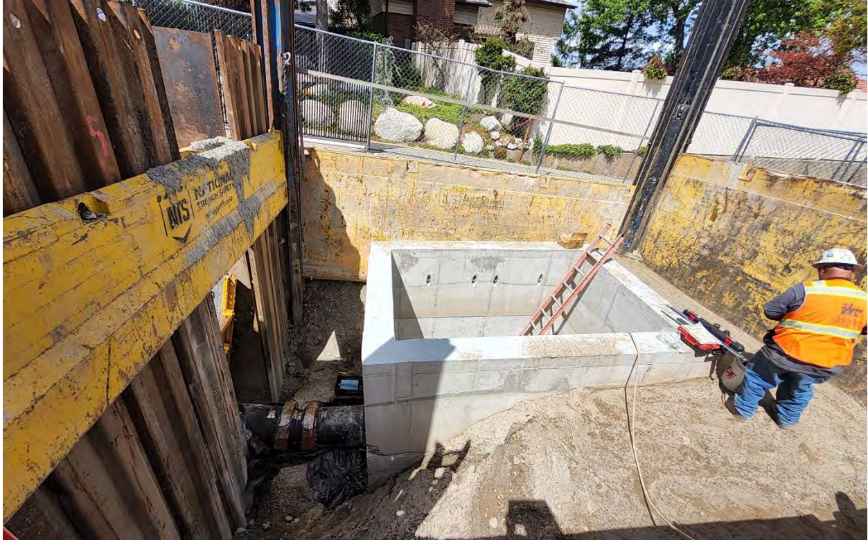
The McEntire Vault was installed in Nutree Dr. This vault includes piping for a future turnout from the SLAR.
