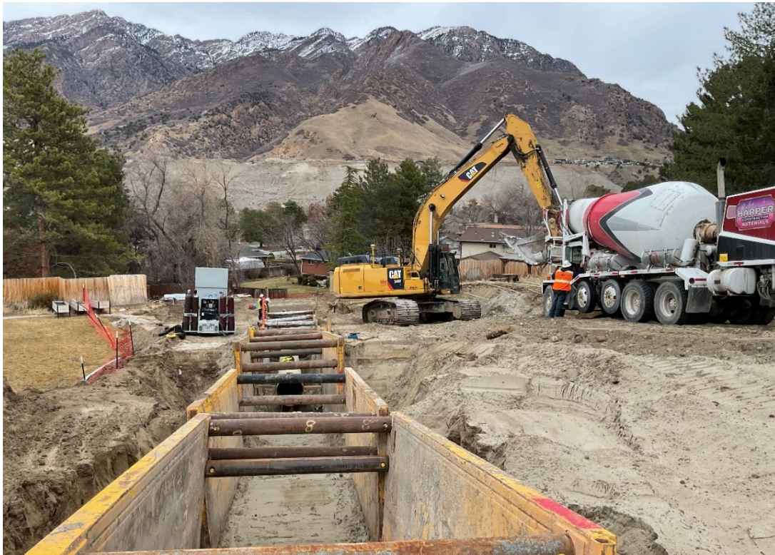
Feb 2: The Little Cottonwood Conduit is being relocated for the new SLAR alignment.
